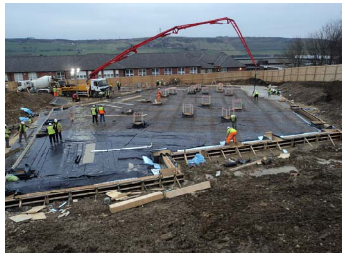
The picture above shows ground workers commencing the first concrete pour, which forms the ground floor slab.
