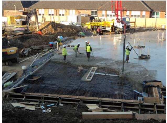
Above shows Operative's levelling the Concrete as It Is poured to form the Ground Floor Slab.
