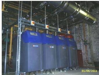
New School Heating Boilers
