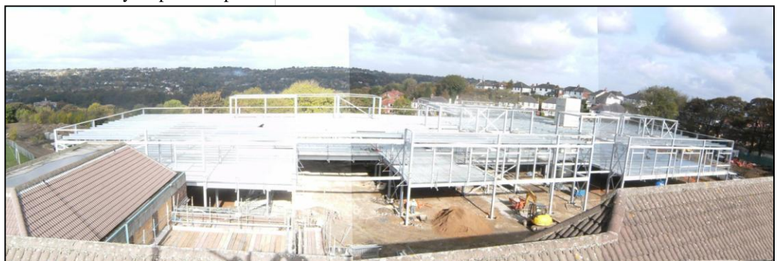
The North Block takes shape with the arrival of the steel framework
