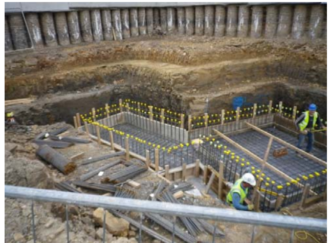
The concrete reinforced foundation is prepared and cast to the biomass bunker located in the 'Energy Centre'.
