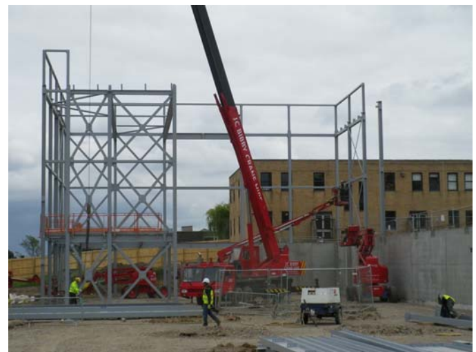
On Monday 11th July the steel frame begins to be erected to the new 'North Block'
