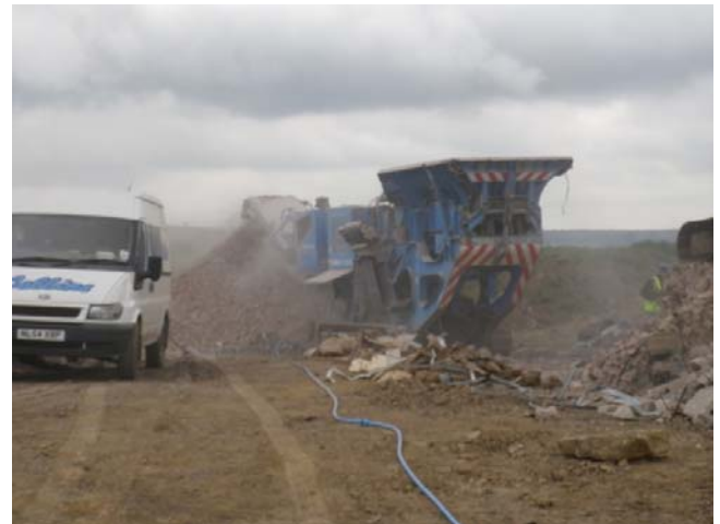
Bricks and concrete foundations from the A3 block remain on site and are crushed to be used as recycled stone on haul roads around site.
